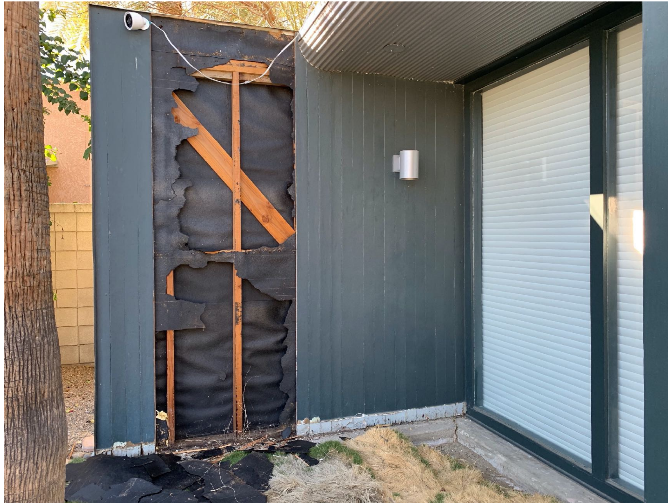
Exterior fin wall off primary bedroom removal and replacement of rotted T&G
