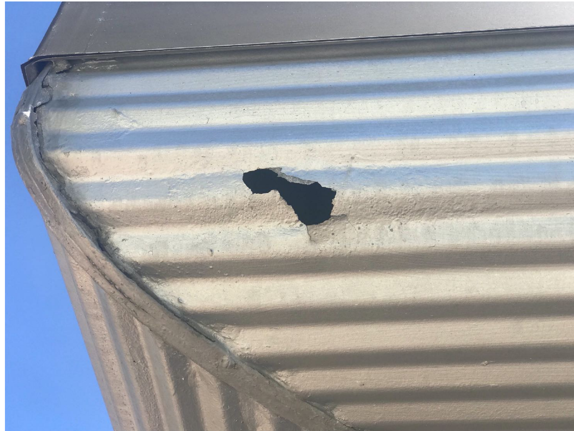
2018 damaged corrugated eaves
