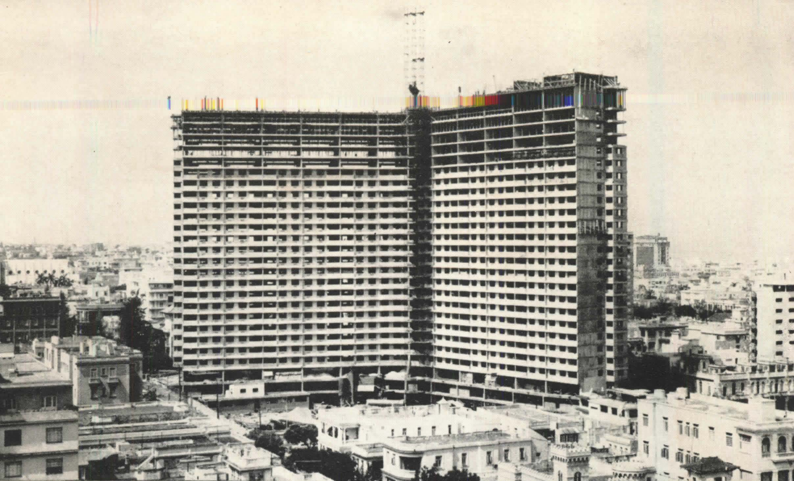
"17 y M"—Reinforced concrete apartment building, Havana, Cuba. Designed to withstand hurricane-force winds. Architect: Ernesto Gomez Sampera and Martin Dominguez; Structural Engineer: Saenz-Cancio-Martin; In charge of Construction: Bartolome Bestard and Manuel Padron.
