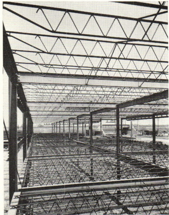
ECONOMICAL through savings in supporting framework and foundations; speed of erection; insurance; maintenance.
