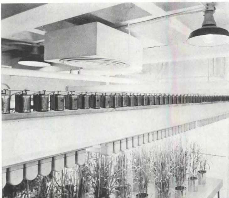
Figure 11—360-cycle capacitor ballasts on fixture in room equipped with high frequency.
