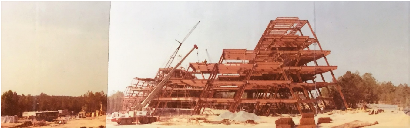
Figure 16: Panoramic construction photograph of the erection of the steel superstructure for the administrative and research wings, circa 1969. Monthly Progress Report, Library of Congress, Paul Rudolph Papers, PR 13 CN 2001: 126, PMR 3042-3.
