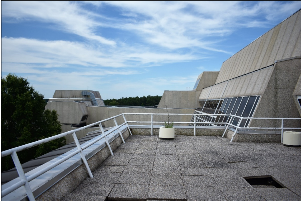
Figure 28: Fifth-level executive terrace, showing original surface treatments, planters, and the deterioration of the foundation. Author's photograph.
